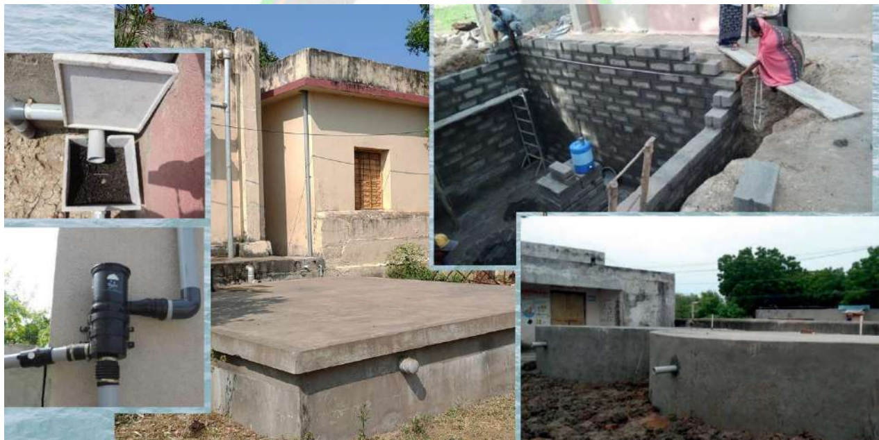
Fig.1: Roof top rain water harvesting
